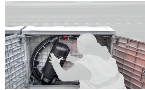
fibre optic cable distributoAr
